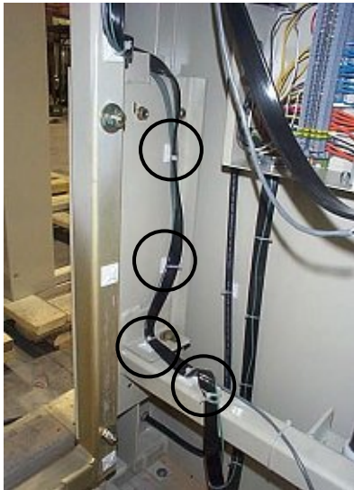
Figure 38 Cut cable ties holding travelling cable
