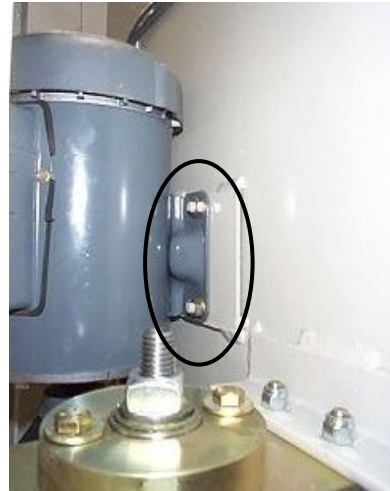
Figure 40 Loosen V-belts by loosening motor base
