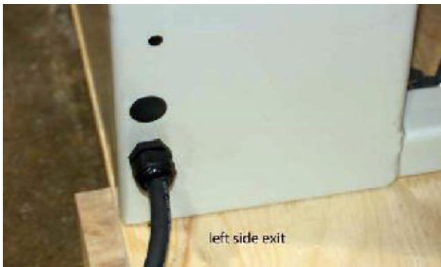
Figure 25 Power cord on left side
